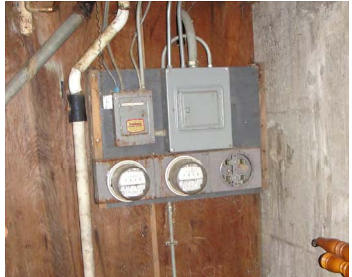
Structural Deficiencies – Outdated and Undersized Systems
