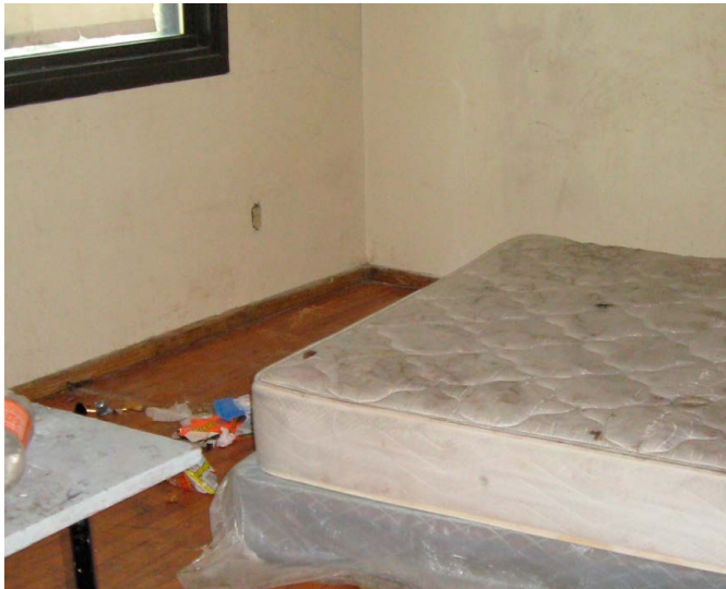
Design Deficiencies - Undersized Rooms Compared to Current Standards
