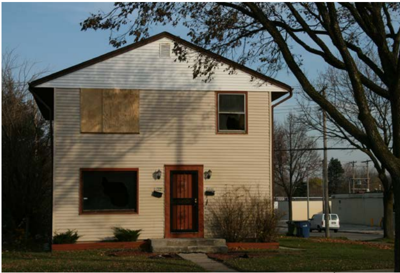
Boarded up house with 2 broken windows (5640-5642 N. 62 nd St.).
