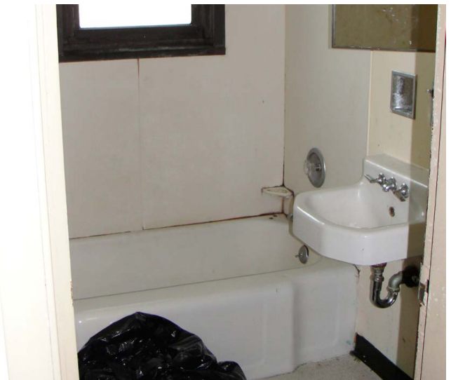
Design Deficiencies - Non-Compliant, Undersized Bathrooms
